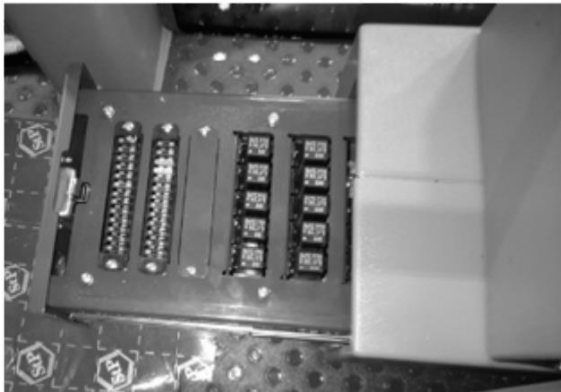
Fig. 1a Switch and protection panel
